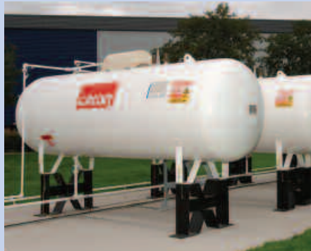
Calor LPG is supplied to each truck via a bulk tank.
